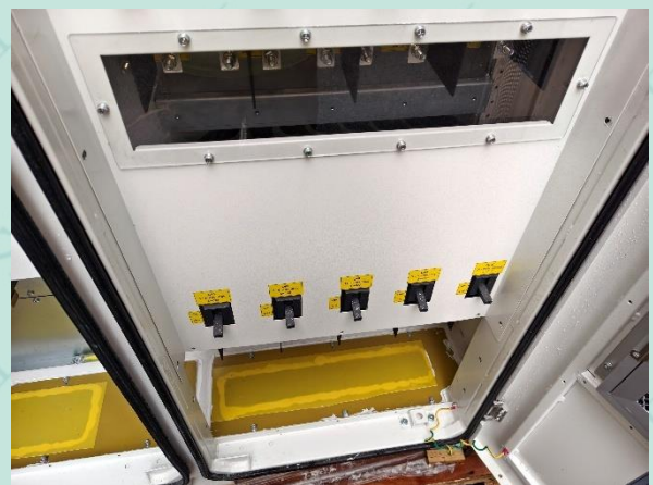
Fig 34 Internal inspection after test
