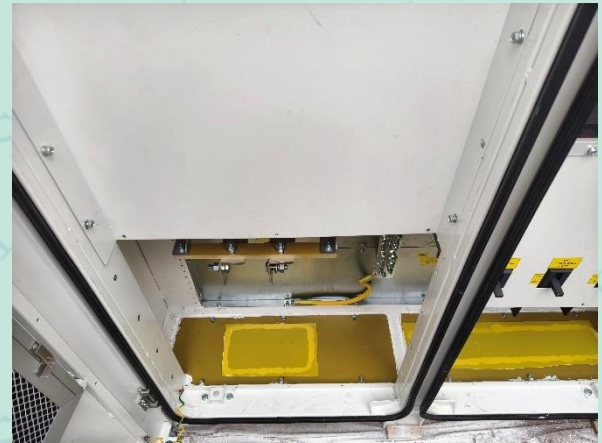
Fig 16 Internal inspection after test
