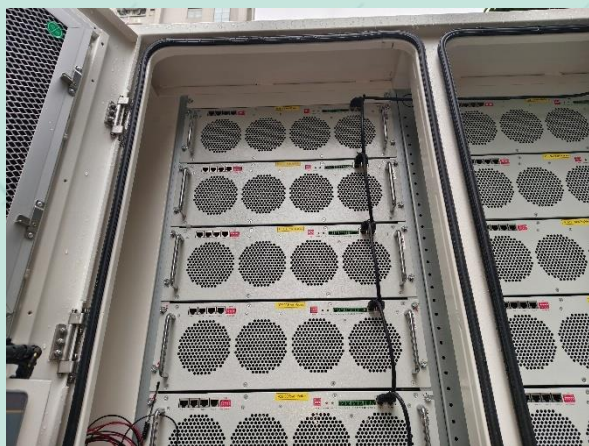
Fig 33 Internal inspection after test
