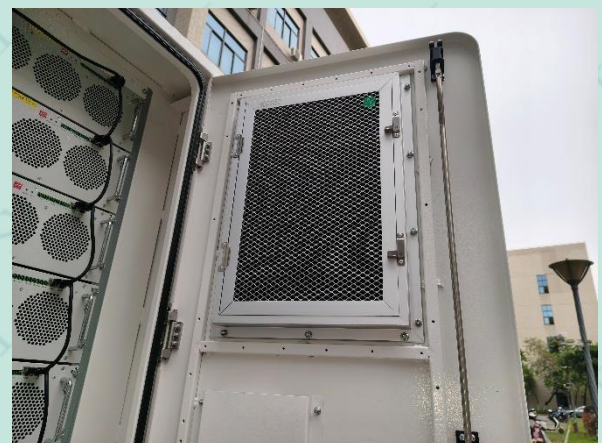
Fig 18 Internal inspection after test
