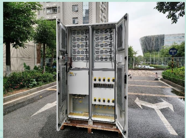
Fig 32 Internal inspection after test
