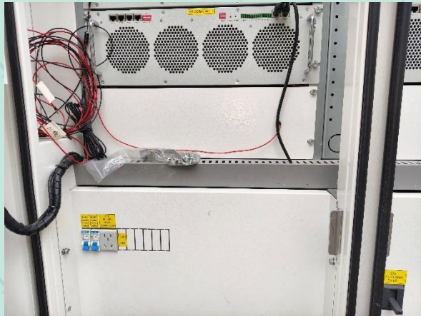
Fig 15 Internal inspection after test
