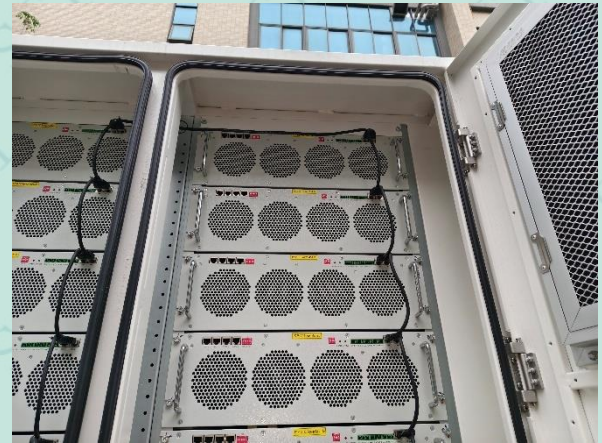
Fig 14 Internal inspection after test
