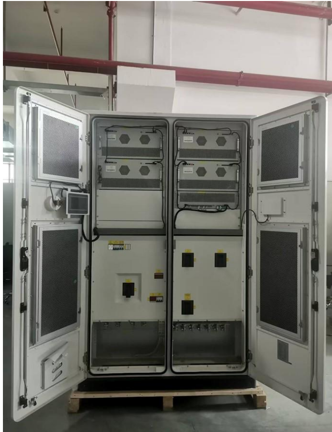
Figure 9 Internal view of Energy Storage Converter (model ESS-GRID P500E)
