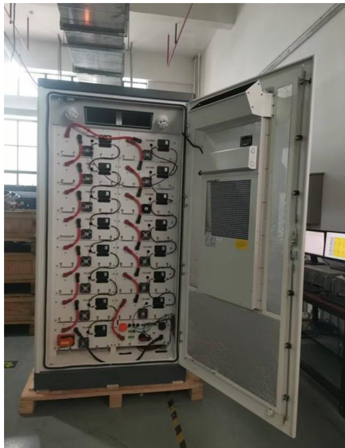
Figure 6 Internal view of Lithium-ion Battery Energy Storage Cabinet
