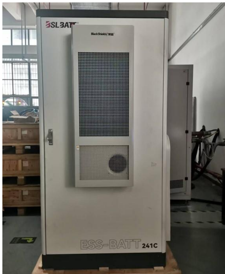
Figure 4 External view of Lithium-ion Battery Energy Storage Cabinet
