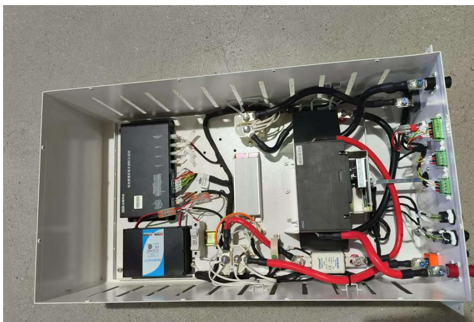
Figure 28. Internal view for High voltage control box
