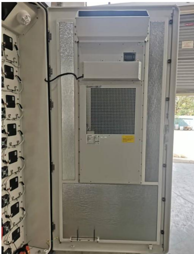
Figure 7. Air Conditioner view
