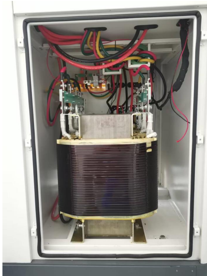
Figure 25. Three-phase isolating transformer view
