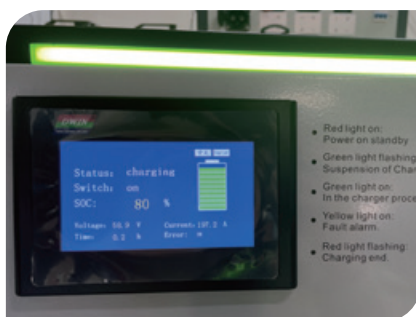
6 观察显示器上有电压与电流，指示灯亮绿灯；表示充电正常 Observe that there is voltage and current on the display, the indicator light is green; it means that the charging is normal position
